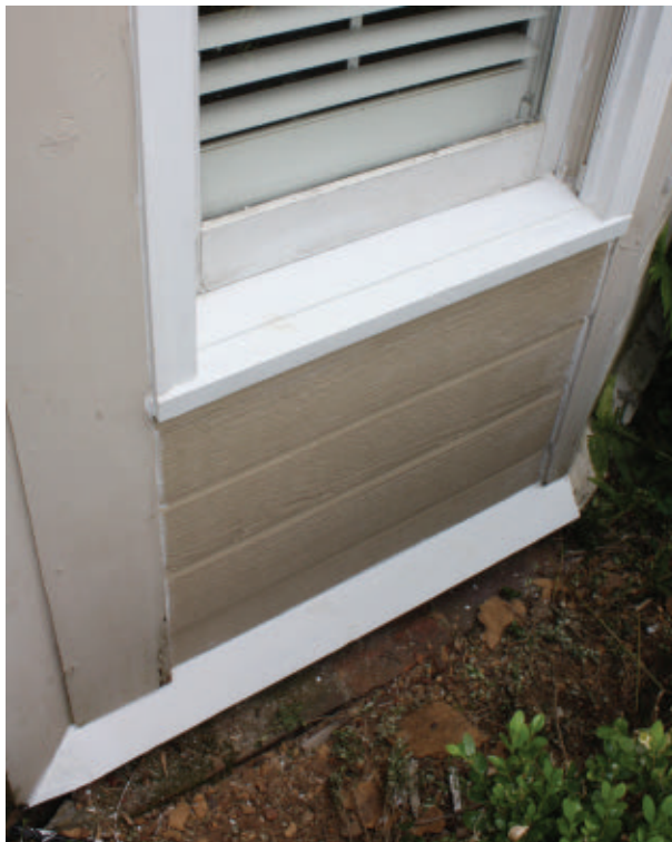
Here's the repair after priming, ready for a new coat of finish paint.
