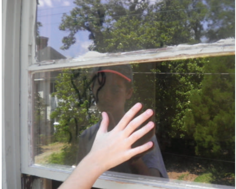
Insert the new pane of glass into the top groove and position it flush against the edges of the bottom and sides.
