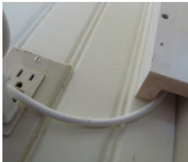
A small, narrow channel conceals the rope lighting as it runs from the outlet to the crown molding.
