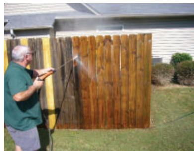
Heavily damaged boards can be completely replaced with new ones, as shown in this photo.
