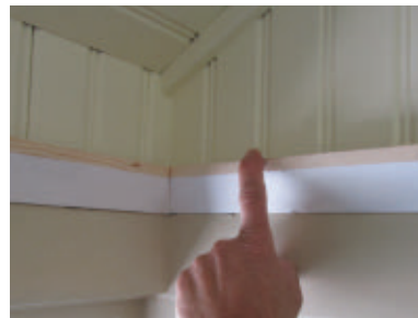
A scrap piece of molding helped to determine the exact corner angles for out-of-square walls.
