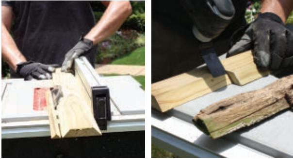
A table saw with a rip fence is the perfect tool for cutting the bevels of the drip edge. A multi-tool made quick work of the notches at the rear of the drip edge.
