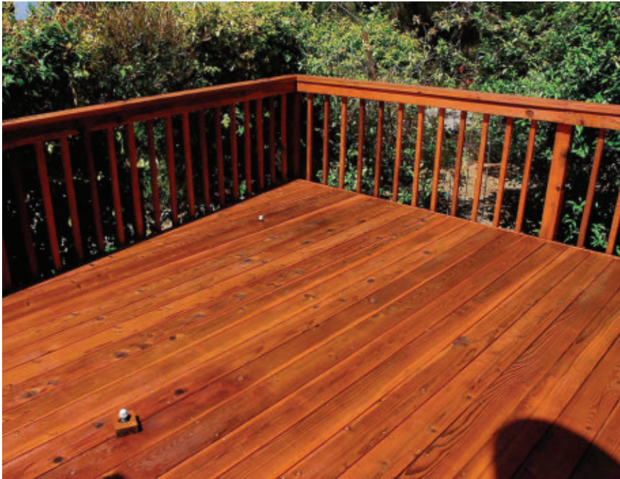
Shown here is the completed deck after proper cleaning, preparation and a new coat of Superdeck.
