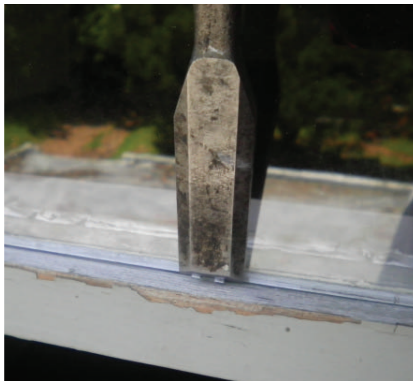
Push the glazier's points into the window frame and then use a flat-blade screwdriver and hammer to gently tap them into place.
