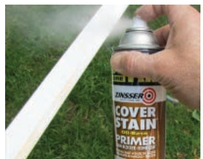
Before installation, all the saw marks were planed off the molding and primer was applied to the exposed wood.
