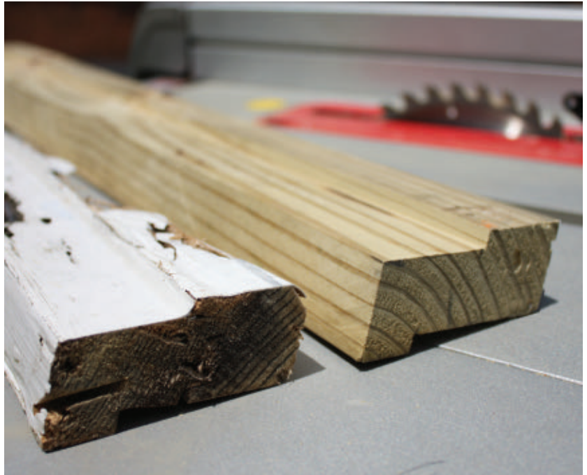
I used the old sill as a template to fabricate a replacement piece on the table saw.
