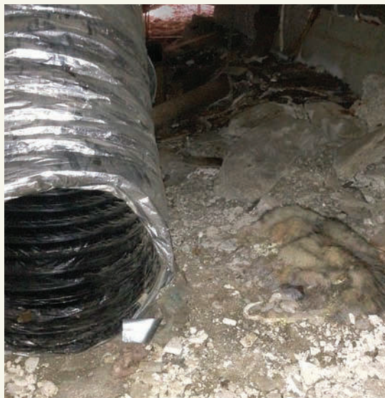
It's what's in the air that matters. A disconnected return duct in most any crawlspace is bad news. In addition to sucking in mold and pesticide residue, this one spices the air with the aroma of dead possum.
