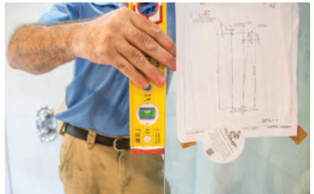
The glass panel is checked for plumb prior to installing the hinged door.
