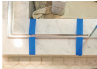
Blue tape holds the U-channel in place during dry fitting and layout.
