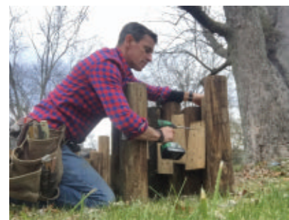
Build the inner circle in two sections. Leave one post out for the hose chase.
