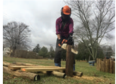
Ripping wedges served two purposes: Secure the landscape fabric and beef up the connections.
