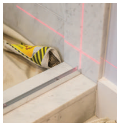
A laser helps to lay out the U-channel and vertical fixed glass panel locations.
