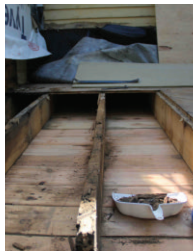
Much of the roof sheathing had also rotted and required removal.
