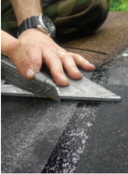
Use a Speed Square as a straight edge for making short cuts with a utility knife around obstacles or to conform to angles that you encounter.
