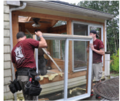
The windows were in good condition to be donated to a Habitat for Humanity ReStore.
