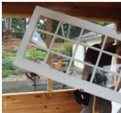
For some exterior doors, only the slab could be salvaged. However, with the interiors we saved the doors and the jambs.
