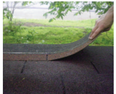
Lay the new starter row of shingles upside-down so the tabs are on the top.
