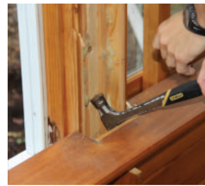
The sill plates were pried away.
