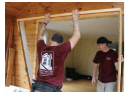
Be careful with the jambs to avoid damage from racking or twisting.
