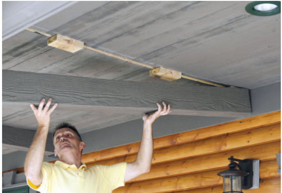
The beams fit over the blocking and fasten in place with a combination of screws and polyurethane construction adhesive.
