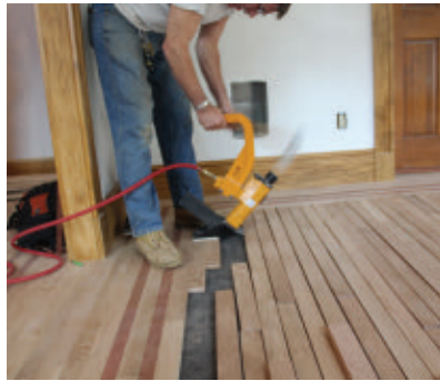
When filling the field of the floor, work from the two opposite longest rows toward the center of the floor.
