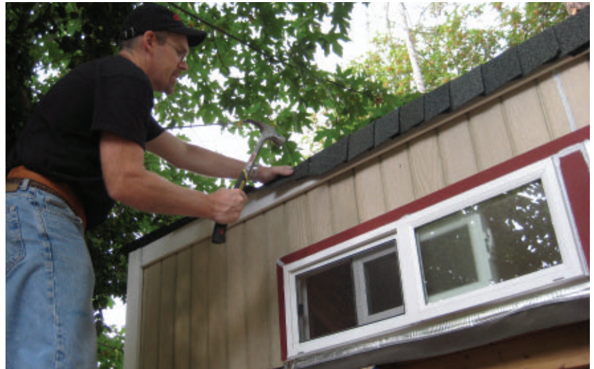
The author installs folded composite shingles opposite the wind direction to finish the front shed roof.
