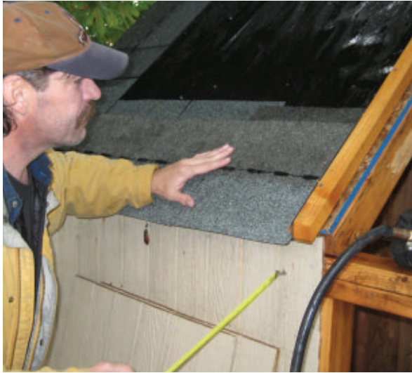
Working through the rain, the author's brother begins the first course on the back shed roof.
