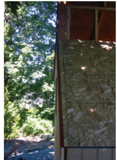
The roofing crew installed filler strips to the skylight roof. Note the mondo gap where the walls meet. Would 1x4 trim be large enough?
