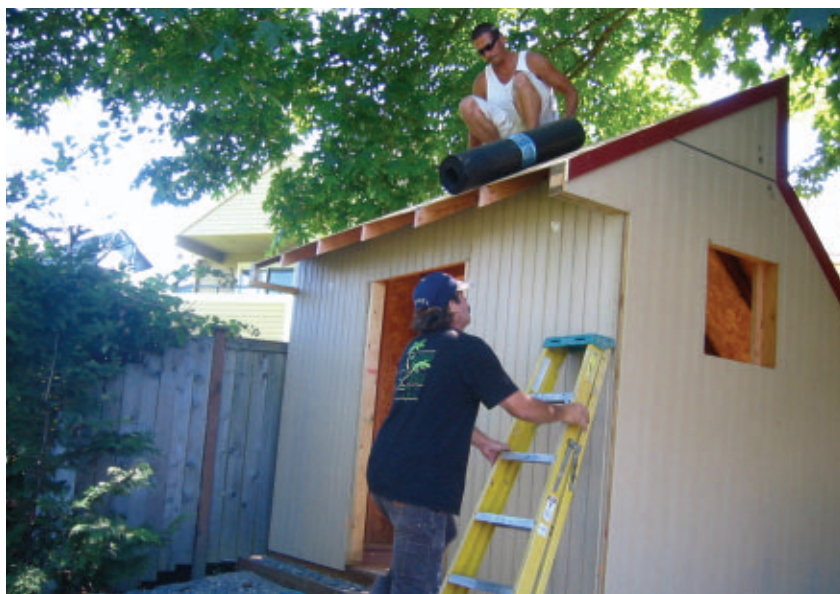
The author's brother (with ladder) and the roofing pro put the lipstick on this pig, four days after their estimated completion. Nonetheless, the shed is starting to look acceptable.
