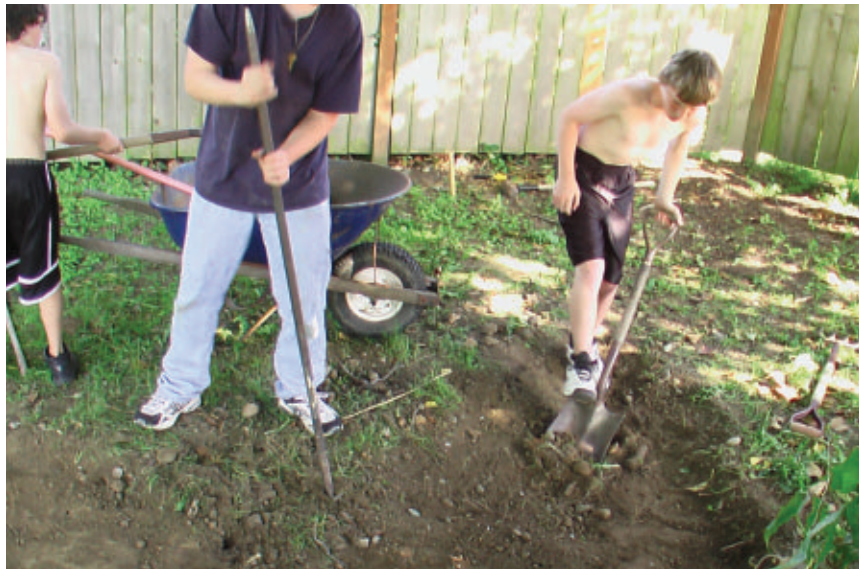
The author's sons and big Mikey (center), dig out the ground for the shed's gravel foundation.
