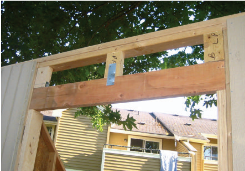
This drop-in header was a marvel of craftsmanship. The cripple studs only vary by 1" from one side to the next.
