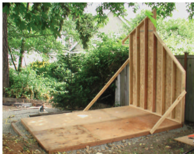
Looking northeast to the left side wall. There was about 18" of clearance between the fence and the eastern wall. It would become a problem during the paint phase.
