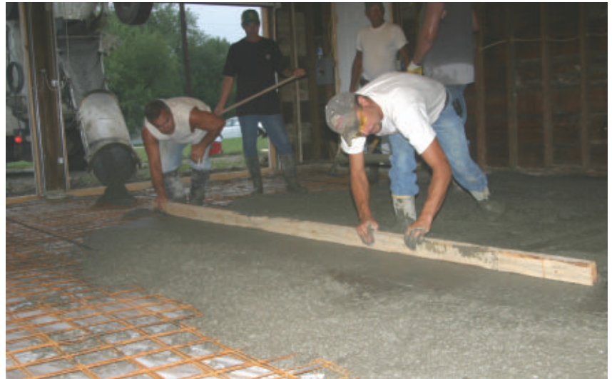
Use a screed board to level the concrete between the forms or guide boards.
