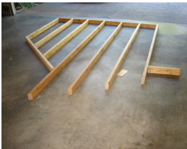
All the wall sections were constructed in the garage starting with the two rake walls. The author used a combination of dimension lumber and LVL studs.
