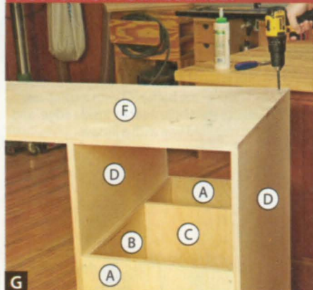
G Flip over the separator box (A–E). Align the end of the separator-box bottom (F) with the outer sides (D) and join with glue and countersunk 1½" screws.
