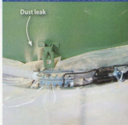
Band clamps don't always form a tight seal when securing a bag, which is usually oversized, to the machine's rim, creating a dust leak under pressure.
