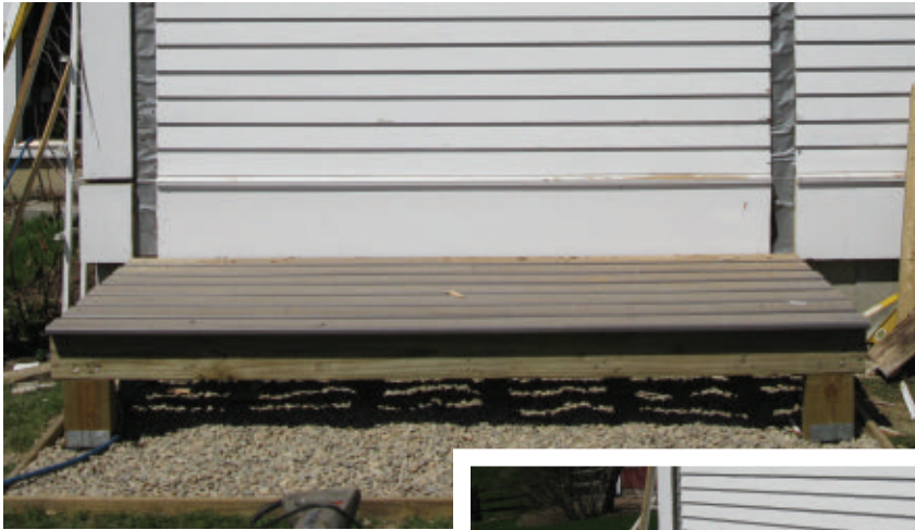
The floor boards were spaced to facilitate air flow to the firewood.
