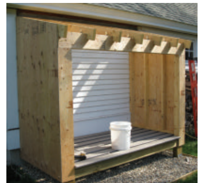
We secured wall and roof sheathing with 8-penny ring-shank nails every 10" in the field and every 6" at seams and edges.
