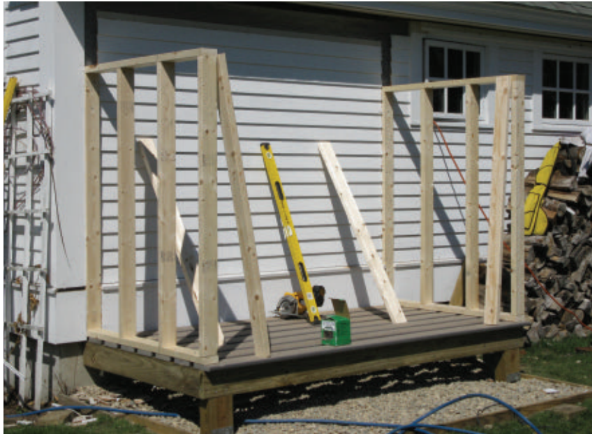
We used regular 2x4 Douglas fir studs 16-in. on center for the wall framing, and built the walls tall enough to accommodate a 3- to 4-pitch roof.
