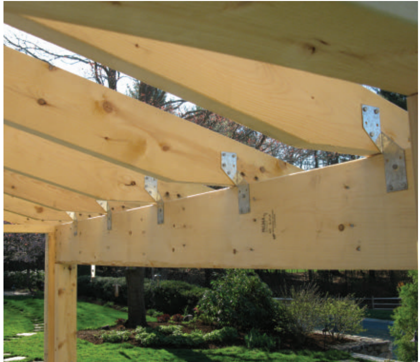
The 2x6 rafters were installed and additionally supported with rafter clips or "hurricane ties".
