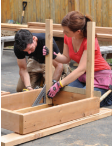
We used a framing square and a layout square to get the staves nice and square.
