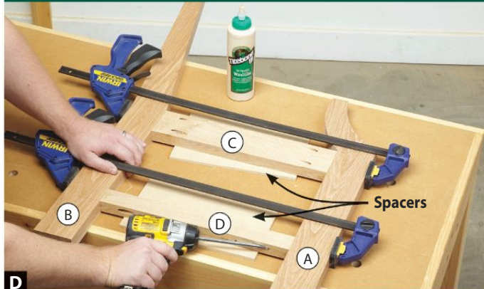
D Rest the side seat rails (C) and side foot rails (D) on \frac{1}{4} " spacers to align them flush with the inside faces of the legs (A, B).
