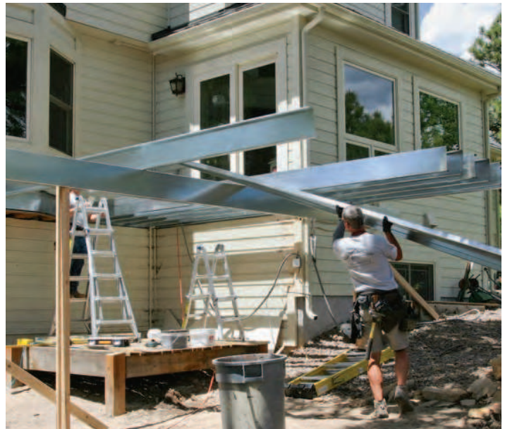
Rust is a reality. Steel deck framing may not rot the way wood can, but it is susceptible to rust and must be coated for protection.
