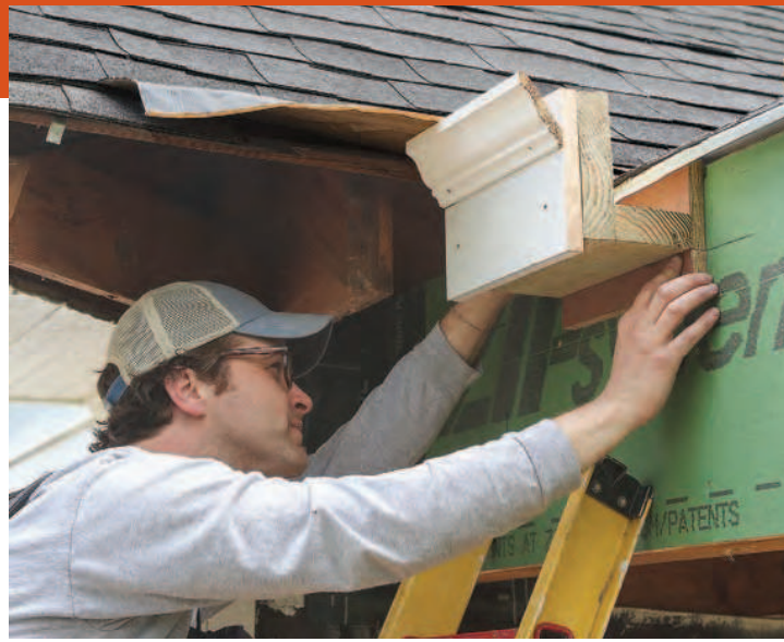
Reality check. Align the cornice mockup so that the bottom edge of the corona framing is set on the datum line to double check that the intended assembly will meet the existing trim. If any components aren't aligned, now is the time to make final changes and compromises.
