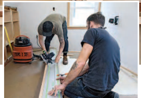
Rip the bevel on the top rail. Using the end stiles that are already fit to the ceiling as a reference, Young rips a bevel along the top rail with a track saw.
