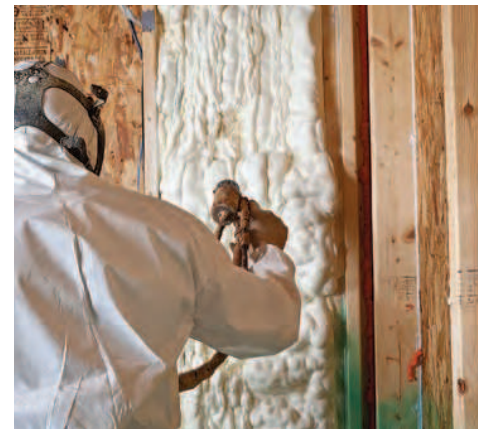
Sprayed and trimmed. Open-cell foam is sprayed to overfill the cavity. After curing, the foam is trimmed flush with the faces of the studs.
