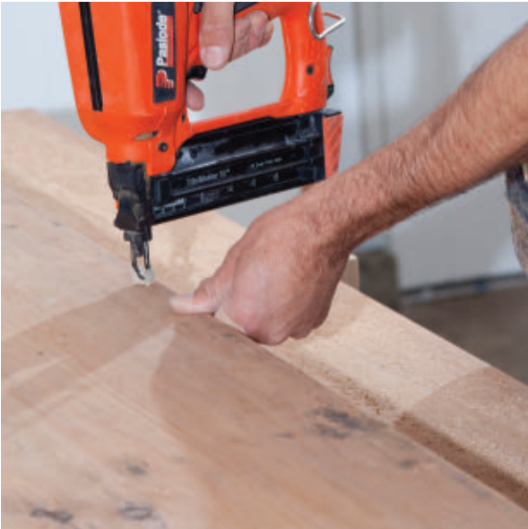
Tack the plywood to the runners in a few places to keep the edges lined up.
