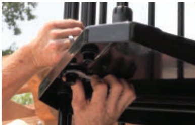
Once in position, the balusters can be secured from beneath the treads.
