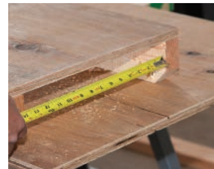
Measure the space between the two table supports and cut wing boards that will fit underneath with about 1/2" of room.
