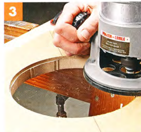
▲ Finally, attach the template to the workpiece with double-sided tape and clean up the hole with a pattern bit.
