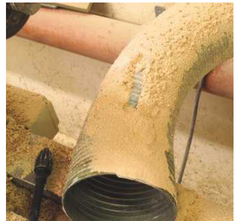
▲ Pic.24 You can see the amount of dust this will create. The 4in pipe cannot cope with these quantities so, as I mentioned earlier, please protect yourself from the dust
