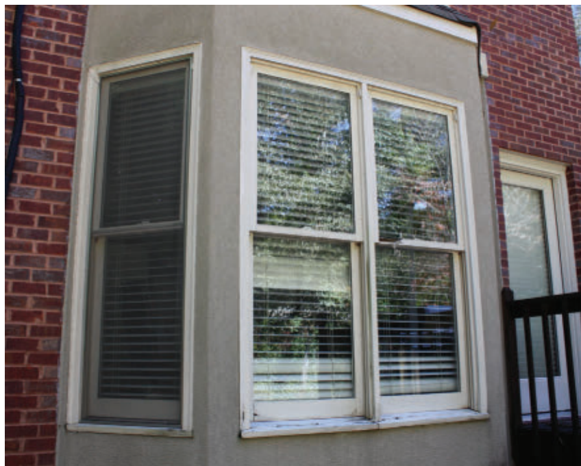
Wood rot is caused by a fungus that thrives on dead wood in moist environments. It can wreak havoc on wood windows.
