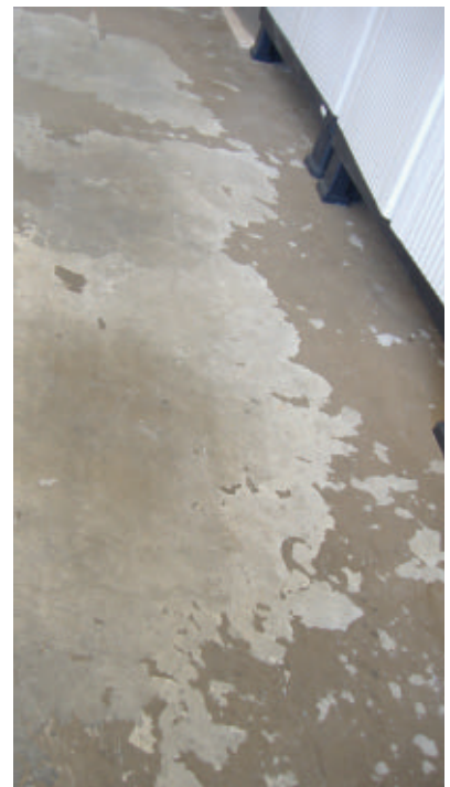
Garage floor coverings can protect the floor and conceal existing damage, stains and concrete discoloration.
