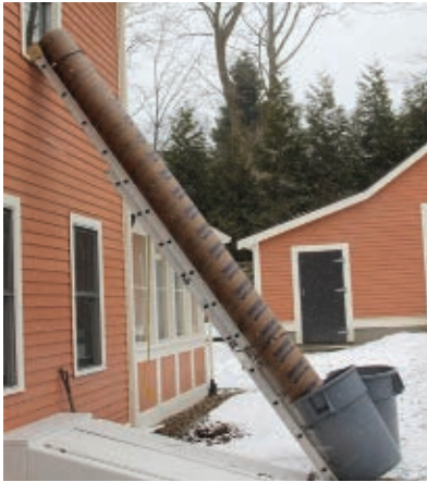
The garbage chute channels demolition debris to a trash can or dumpster on the ground.
