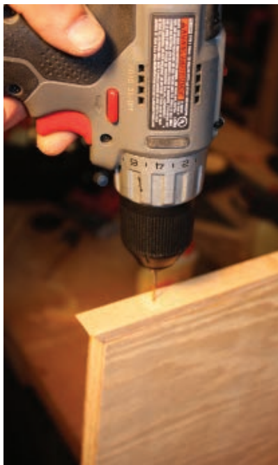
The edging was installed with a combination of wood glue and finish nails, with holes predrilled for the nails.
