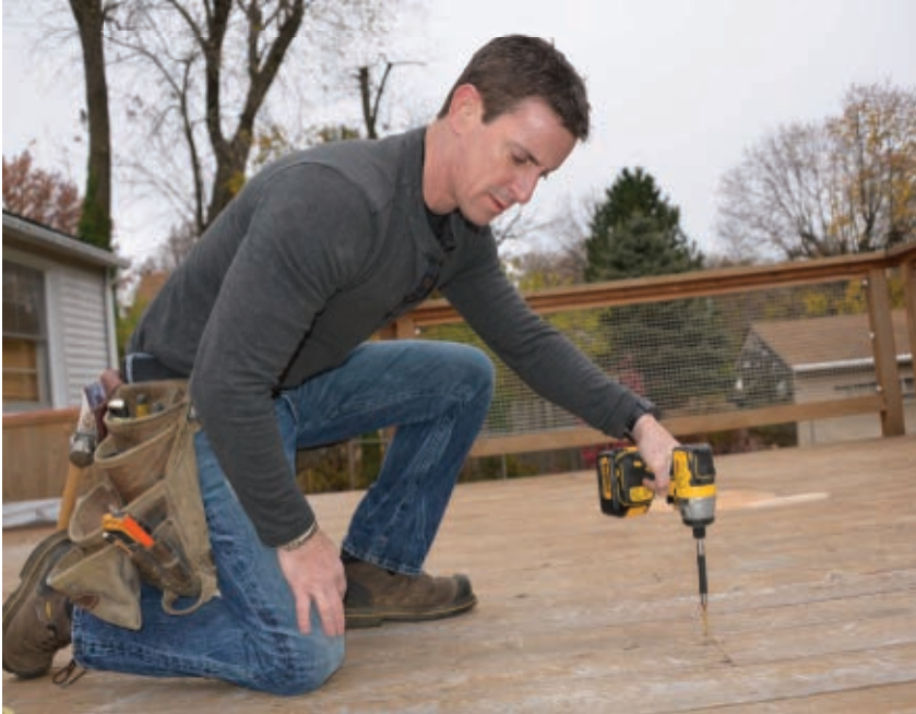
An important first step in deck maintenance is to check each fastener to be sure none are coming loose.
