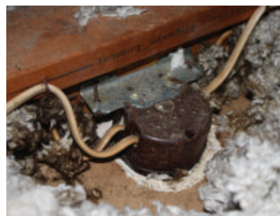
Inside the attic I found the old outlet box buried beneath loose insulation attached to the side of a ceiling joist.
