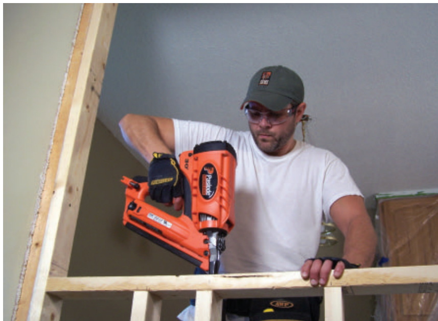
I then nailed the top plate of the bar in place and installed the cripple studs flush beneath it.
