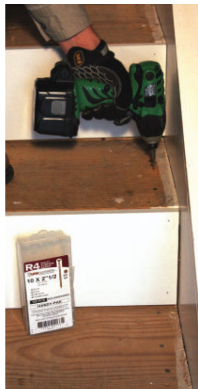
Screw down the existing treads into the stringers to eliminate any squeaks.
