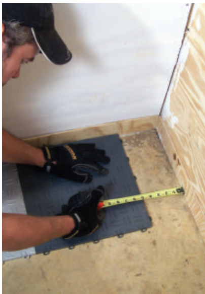
For a symmetrical layout, center the first row and cut partial tiles for each end.
