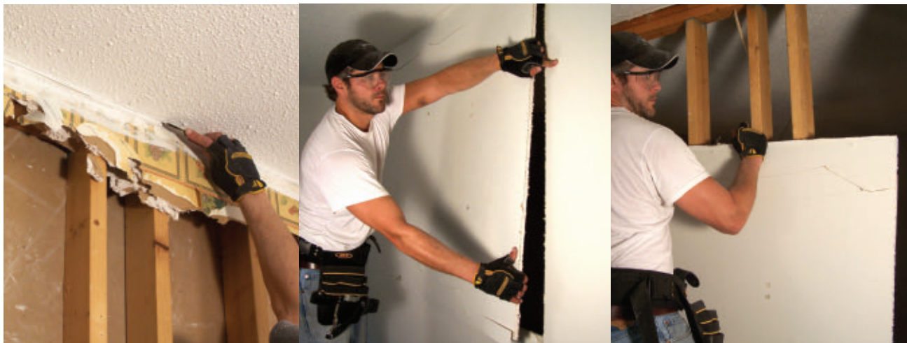
Cut the drywall joint so it separates from the ceiling without damage.
