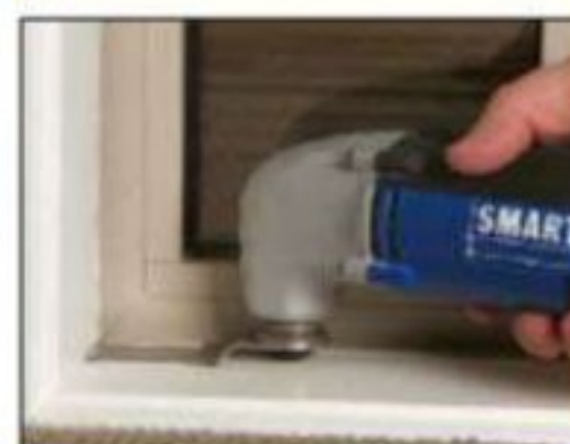
UNDER CUTTING DOOR JAMBS
