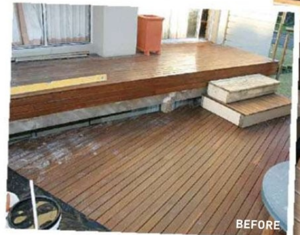
The narrow steps that joined the split decks gave limited and inconvenient access.
