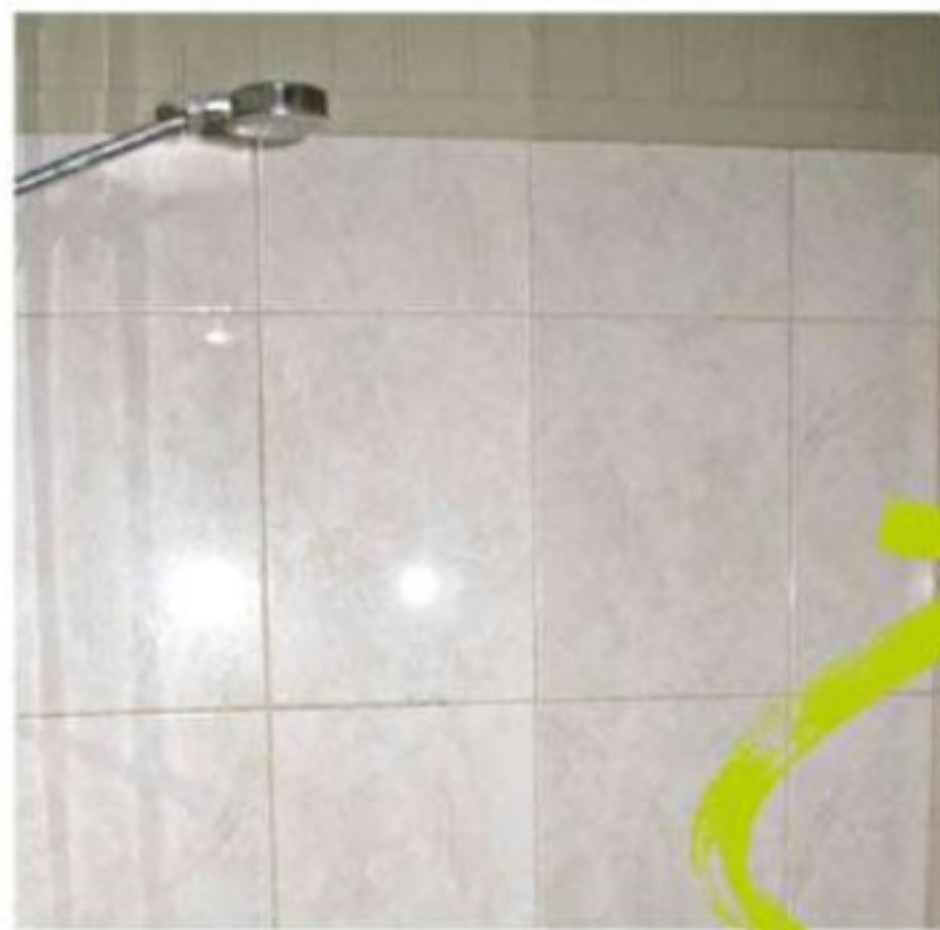
Tank water had discoloured the tile grout in the shower recess.
