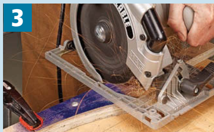
3 Score Centerline. I used an inexpensive abrasive blade in the circular saw to cut just over halfway through the brace.
