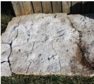
After 24 hours, the slab was webbed with cracks.
