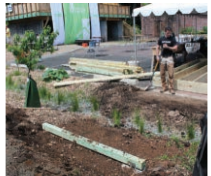
We installed a 4x4 grade beam and LedgerLOKed our bridge to it. This helped us set the structure to minimize digging.
