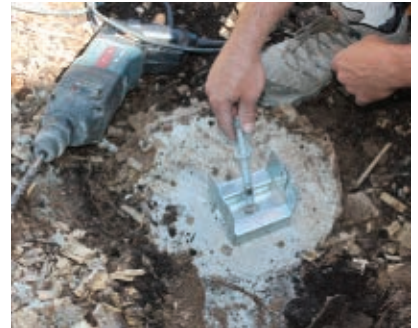
Forget J-bolts and wet concrete. We let the posts cure, then Bosch Bulldogged some 1/2" holes for galvanized Red Head sleeve anchors.
