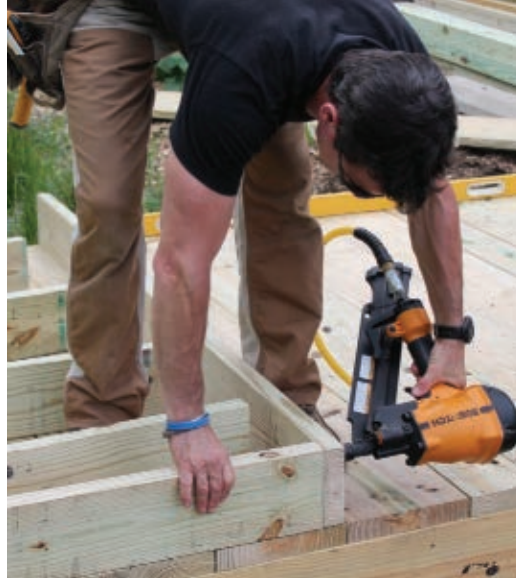
We built a smaller bridge box to extend the bridge to its termination point at grade.
