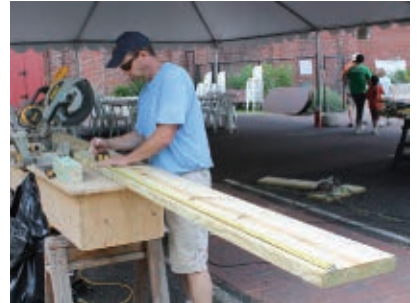
Pre-cut 10' deck boards in half on the miter saw, then run the ends wild before cutting all at once in place.
