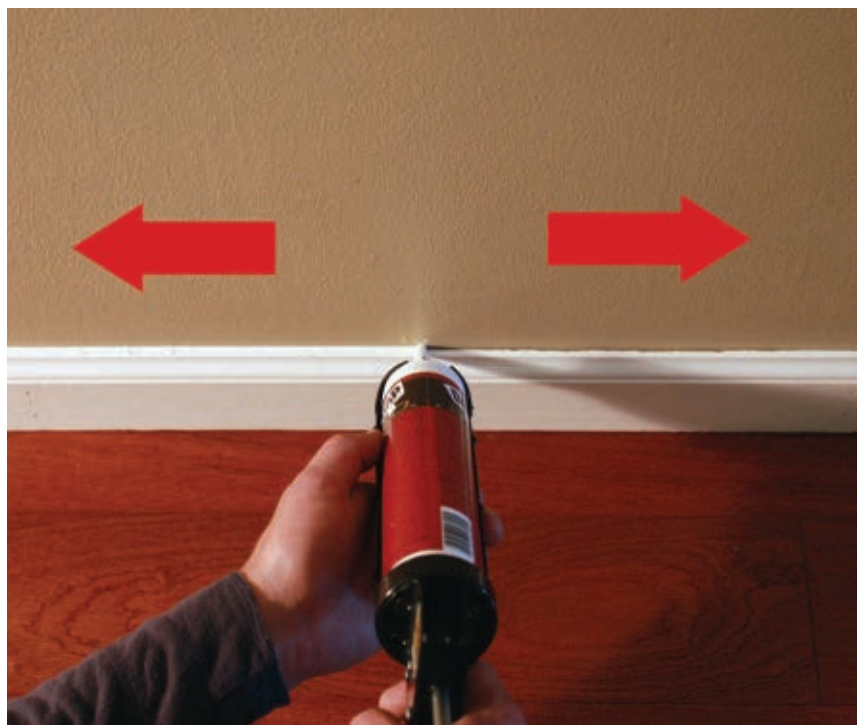
Hold the gun at a right angle to the joint as you lay the caulk bead. The right-angle position strikes a balance between pushing and pulling for consistent application and easy visibility on both sides of the nozzle.
