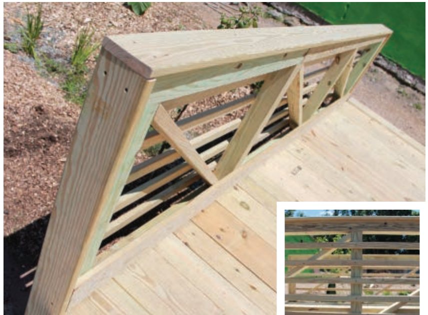
4x4 trim, horizontal rails, 2x4 diagonals and a 5/4 wrap add character and “space” without over-detailing it.
