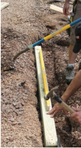
We built a "pad" with pea gravel and a second 4x4 grade beam to support the bridge extension.
